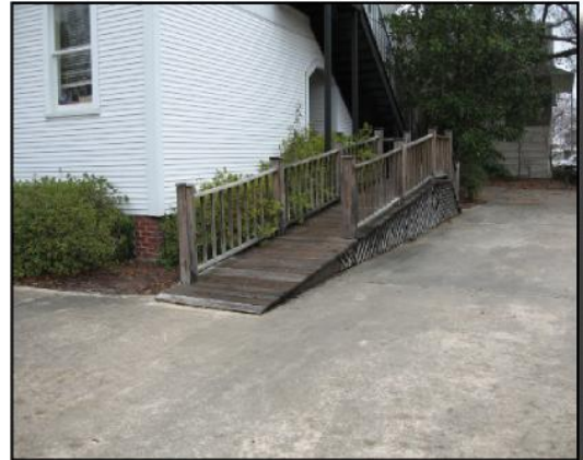
Handicapped ramps should be sited on the side or rear rather than on the front of dwellings.
