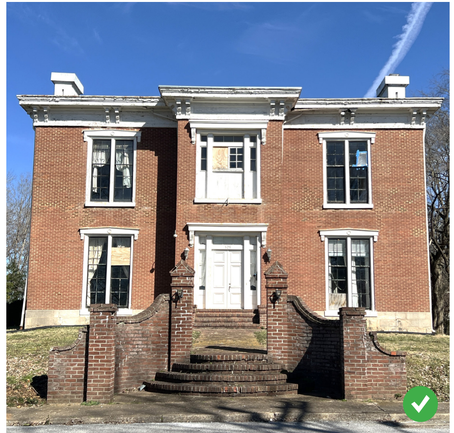
Although this brick entrance treatment on York Street appears to date from after the antebellum era of its associated house, it is still historic and important to preserve.
