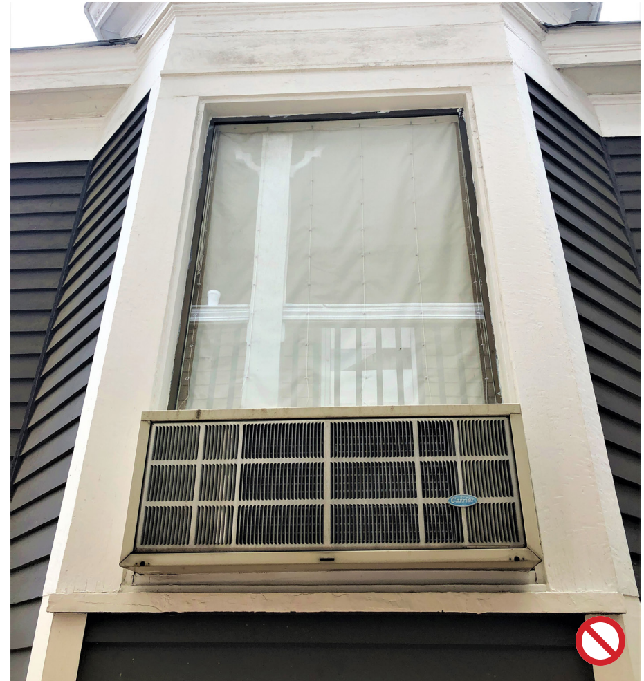
Air conditioning units should be avoided when possible, particularly on front facades.
