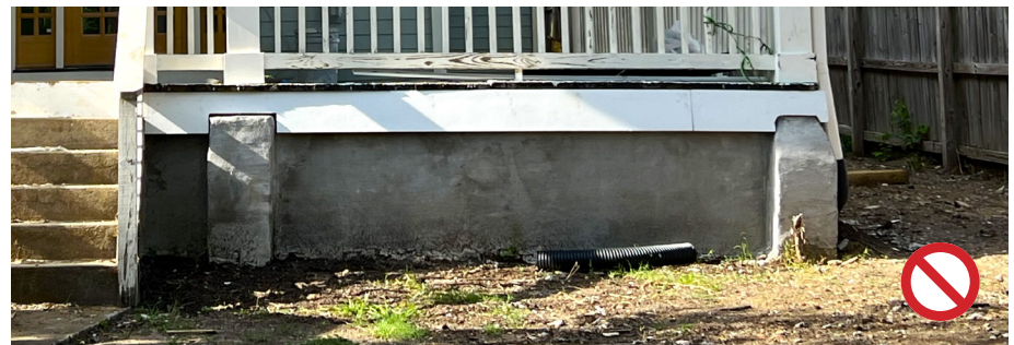
This house's brick foundations have been parged with concrete, which alters the historic appearance and traps in moisture that can lead to future deterioration.
