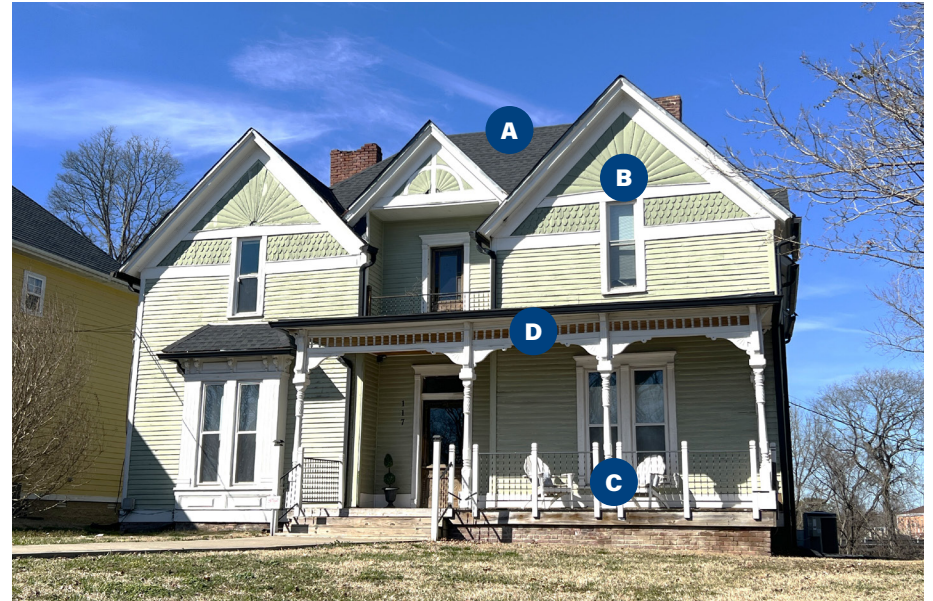
This two-story Queen Anne style house in the Emerald Hill Historic District is a fine example of this style of architecture. The only exception is the replaced hand rails on the porch and recessed balcony.
