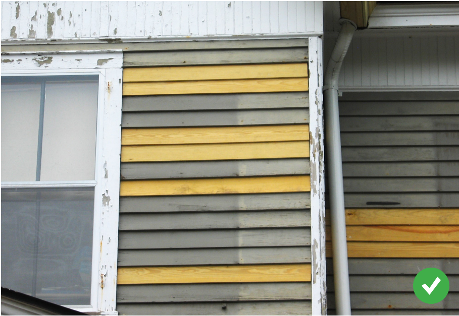
Although this exterior wall still needs repainting, these new clapboards match the originals with respect to their exposure width and other characteristics
