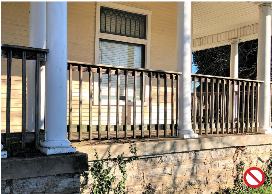
This is an example of inappropriate porch railings on a historic home located in another community.
