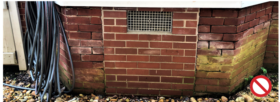
The design of the brick infill between the historic brick piers is inappropriate.
