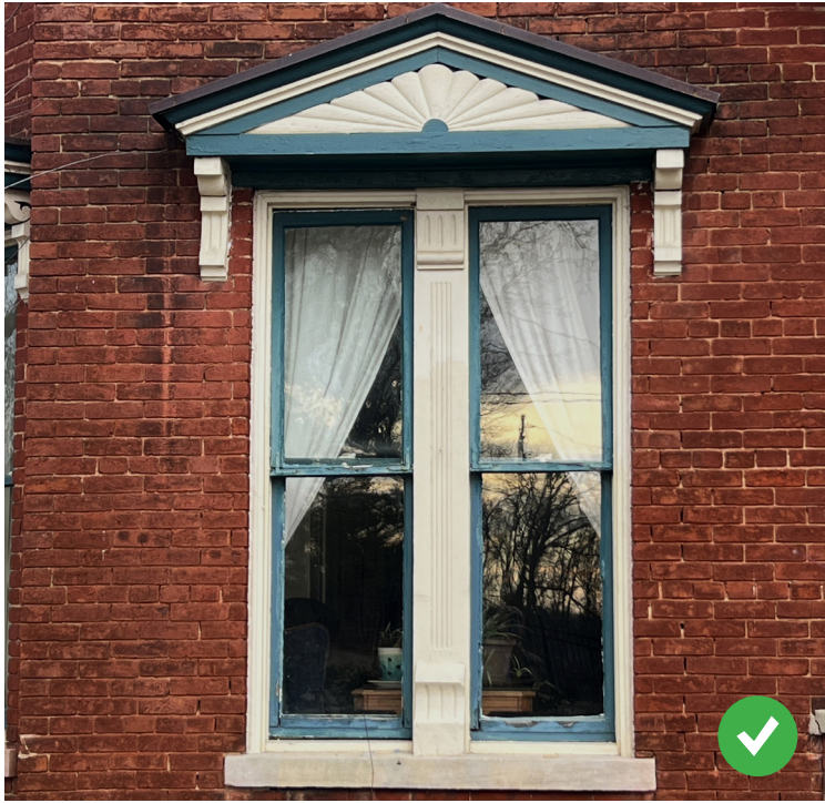
This window is on the front facade of a brick Queen Anne style house in the Dog Hill Historic District. This original window features paired one-over-one double hung windows.
